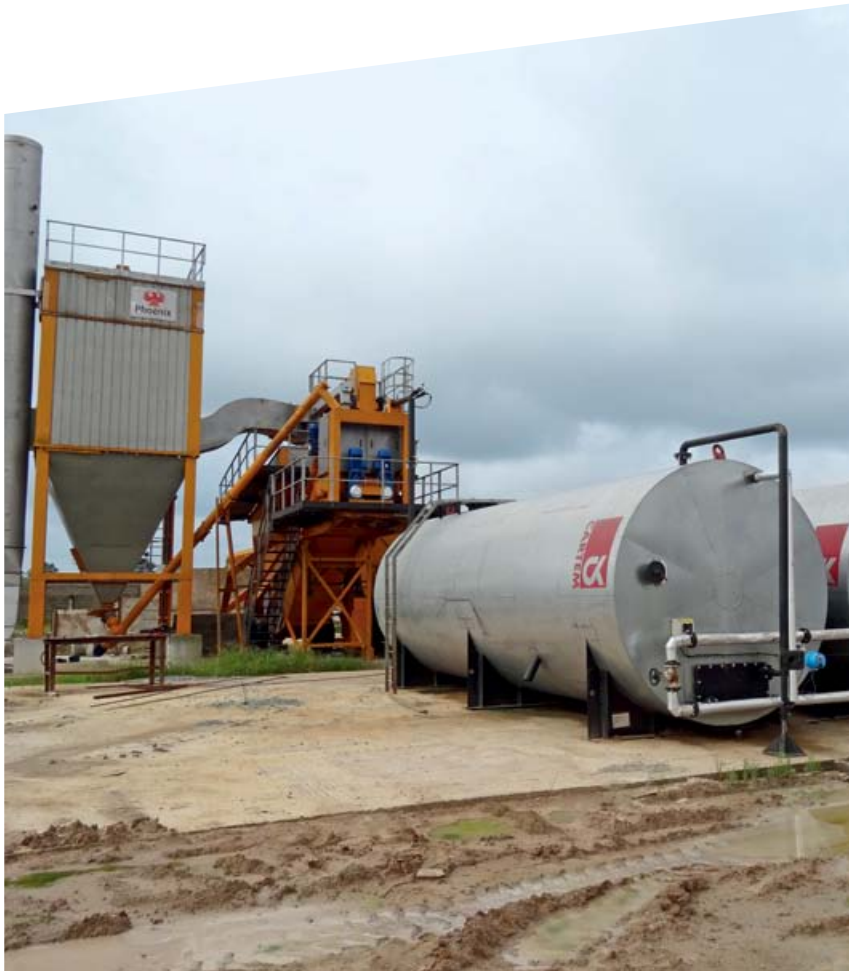
••• Production of asphalt mixtures - asphalt Batching plant.
