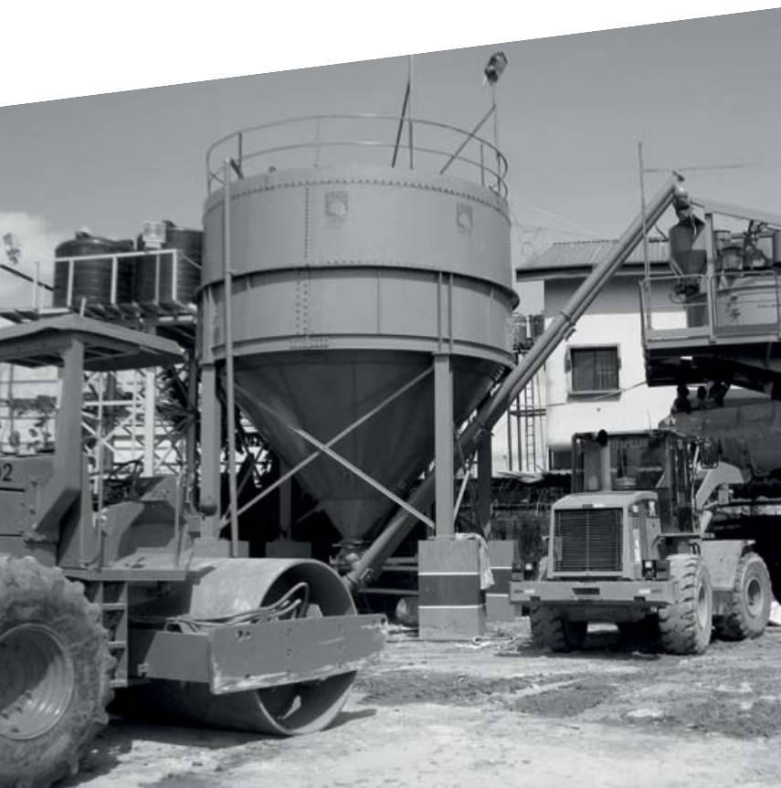
••• Precast yards producing precast concrete elements such as medians, drainages, channels, manholes and kerbs for road infrastructure.
